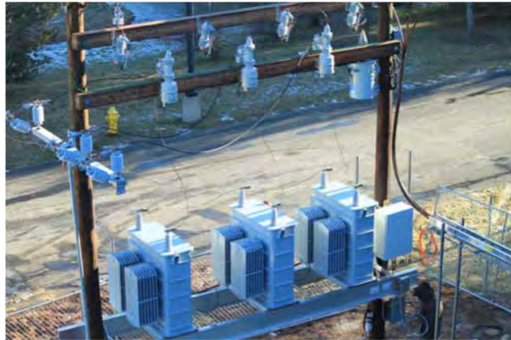
Example of an above ground feeder installation
