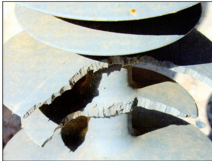
Figure 6.4: Example of rodent attack on the silicone sheds [6.1]
