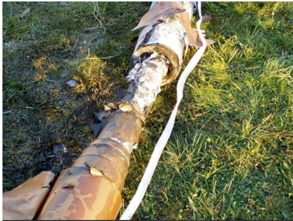
Figure 4.1.3.3: Axial destruction of OIP bushing (layer sliding) probably because of poor paper sheet overlapping
