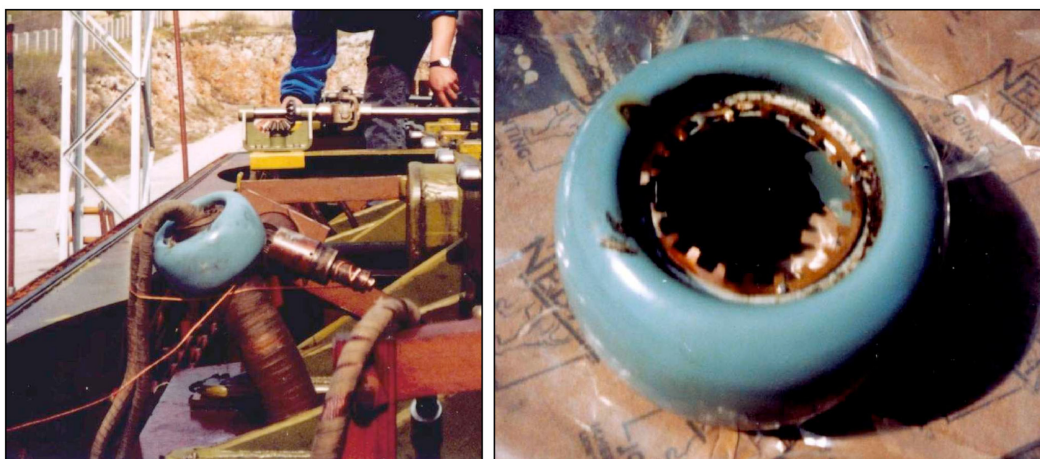
Figure 4.1.3.13: 245 kV bushing end shield fallen down (left), low energy arc traces on the shield (right)
