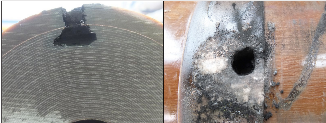
Figure 4.1.3.10: Test tap problem that penetrated deeply into the RIP body possibly caused by VFT (left core cut view, right: damaged test tap)
