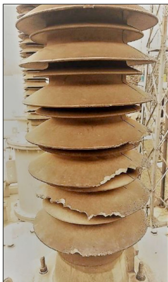
Figure 4.1.4.4: In-service bushing's silicon sheds attacked by monkeys [3.2.8]
