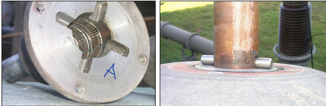
Figure 5.2.4.1: Overheating traces on a 220 kV bushing upper connection (left: on the multi-contacts and upper aluminium connection, right: on copper bolt above bushing head)
