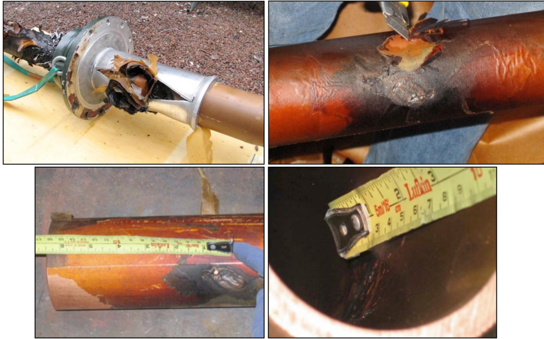
Figure 4.1.2.2: 700 kV transformer failure; top left: 300 kV failed bushing, top right: intensive thermal degradation of paper near central tube, bottom: breakdown traces on the outer side of central tube (left) corresponds to arc traces on the inner side of the tube
