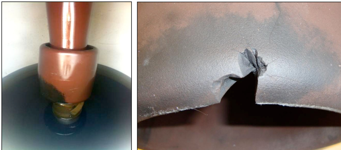
Figure 4.1.3.14: Two examples of similar cases showing end shield electrical problems: breakdown traces on 420 kV bushing end shield in turret (left), detail of end shield resin rupture after breakdown (right)
