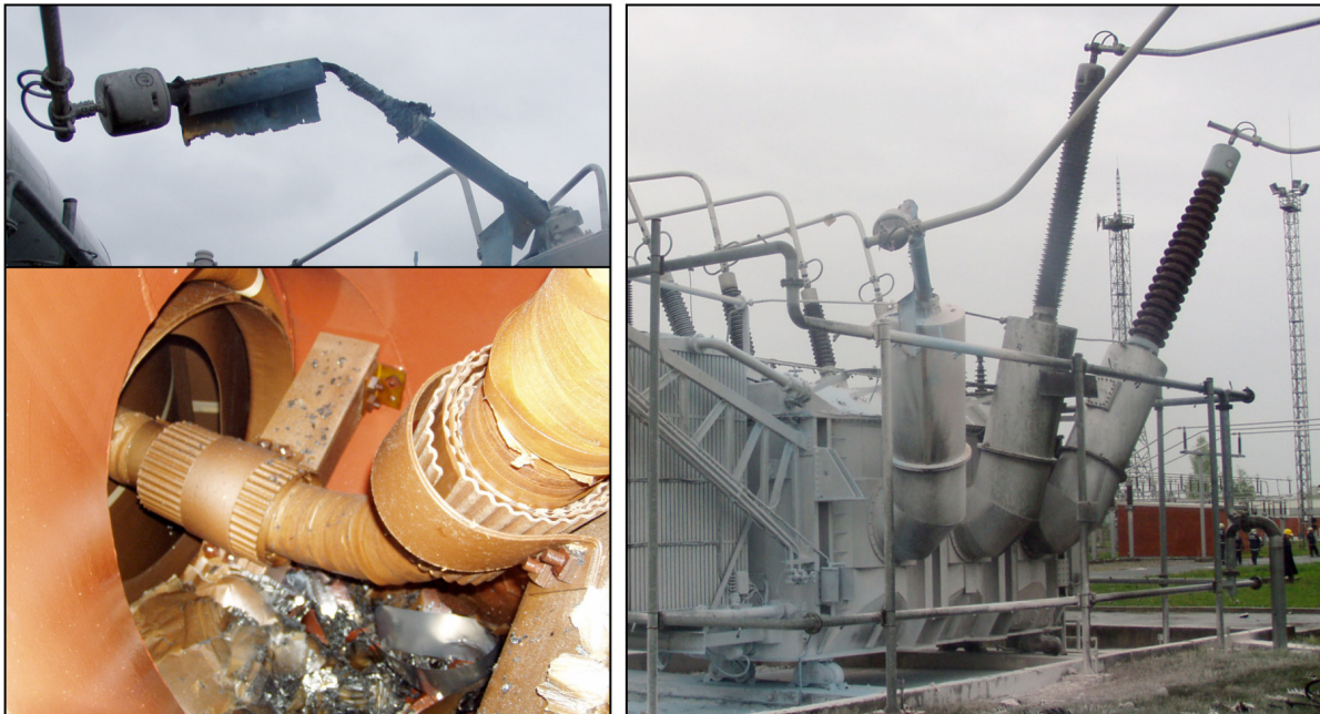
Figure 3.1: 400 kV failed bushing (up, left) and fire at 300 MVA transformer (right); bushing fragments in transformer turret and tank (down, left)
