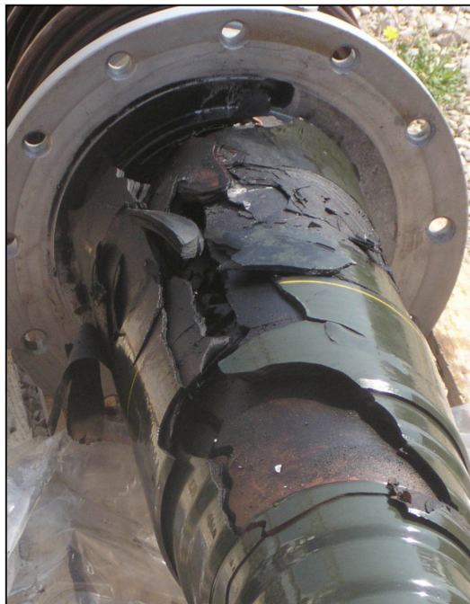
Figure 4.3.1: Exploded oil part of 30 years old, 245 kV, RBP bushing
